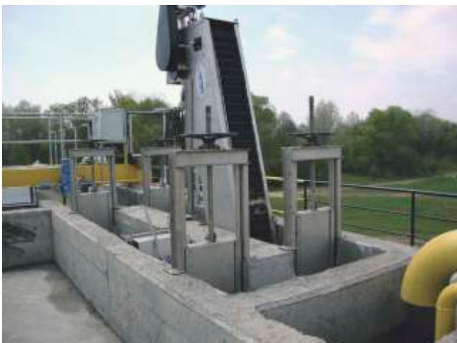
Evsel Atıksu Arıtma Domestic Wastewater Treatment
